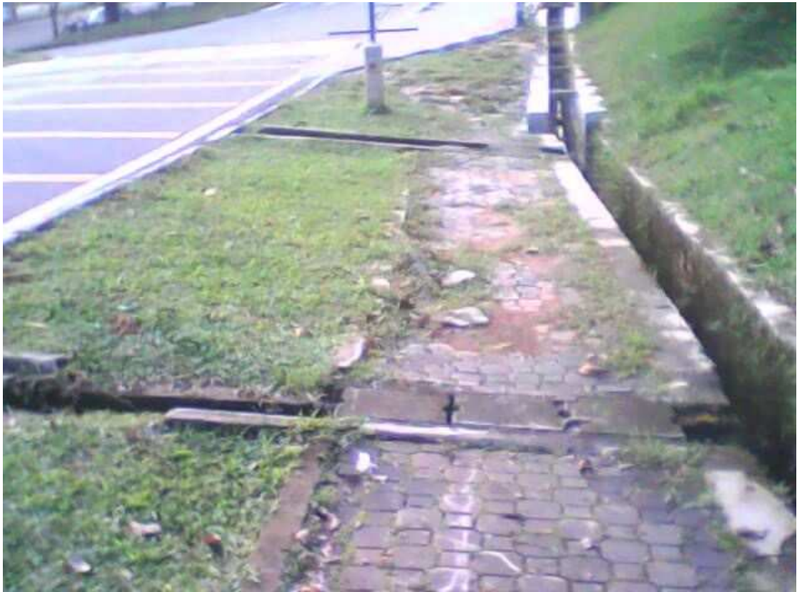
Figure 1-3 Dilapidated NMT facility opposite Block B11
