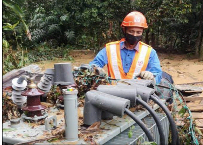
Figure 1.2 Example of the grid utility power distribution equipment affected due to severe flood disaster. (This photo is obtained from [10])
