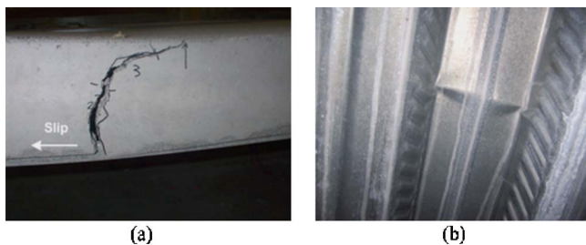
Fig. 7. (a) Major crack due to horizontal slip failure; (b) buckling of deck top flange
