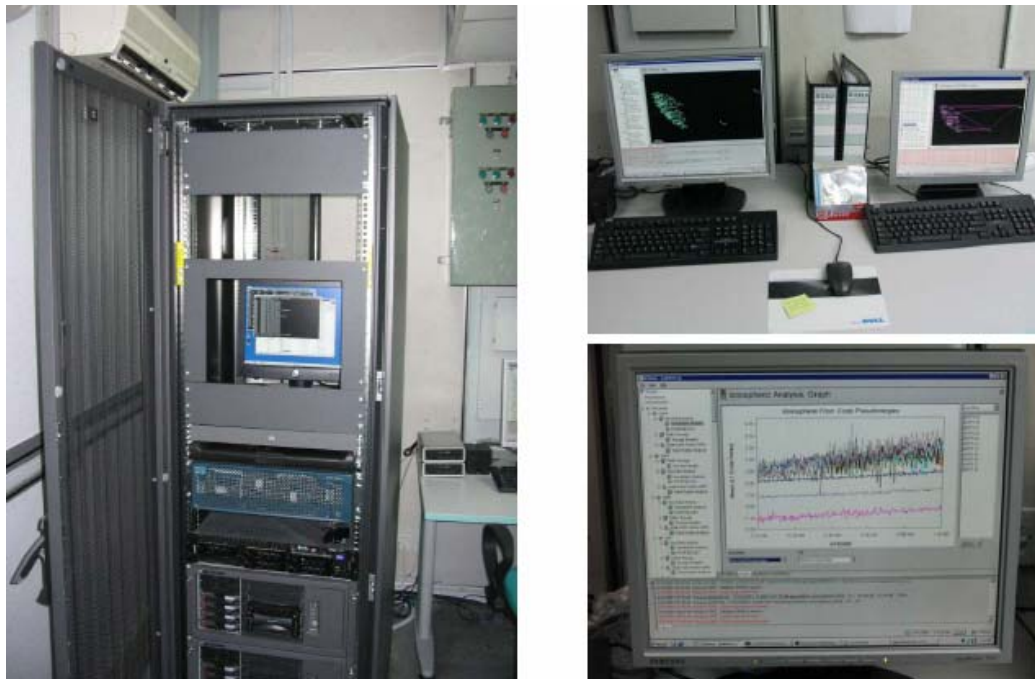
Figure 3.19: MyRTKnet Control Centre and Equipment
