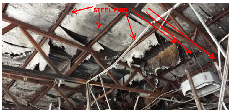
Figure 4. Observation on steel purlins that were affected by fire.
