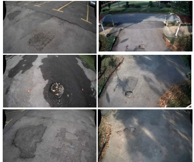
FIGURE 9. Sample images for road damage.
