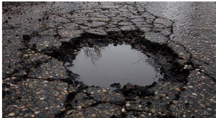
Figure 1. Pothole on the road.
