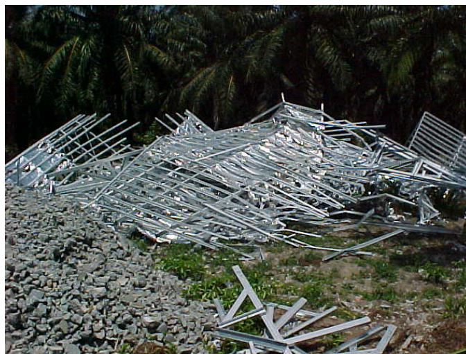
Figure 1.1: Cold Formed Structure under Failure
