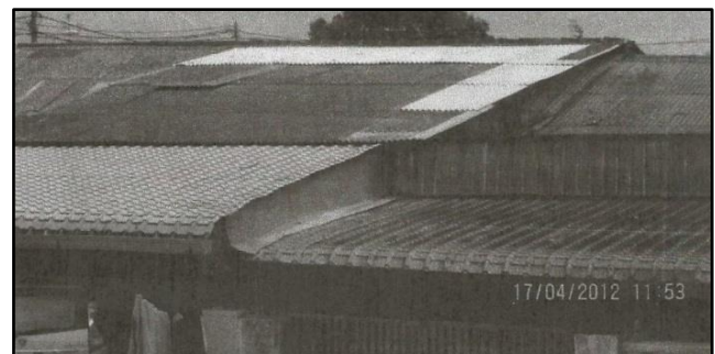
Figure 3. Damages that have been repaired
