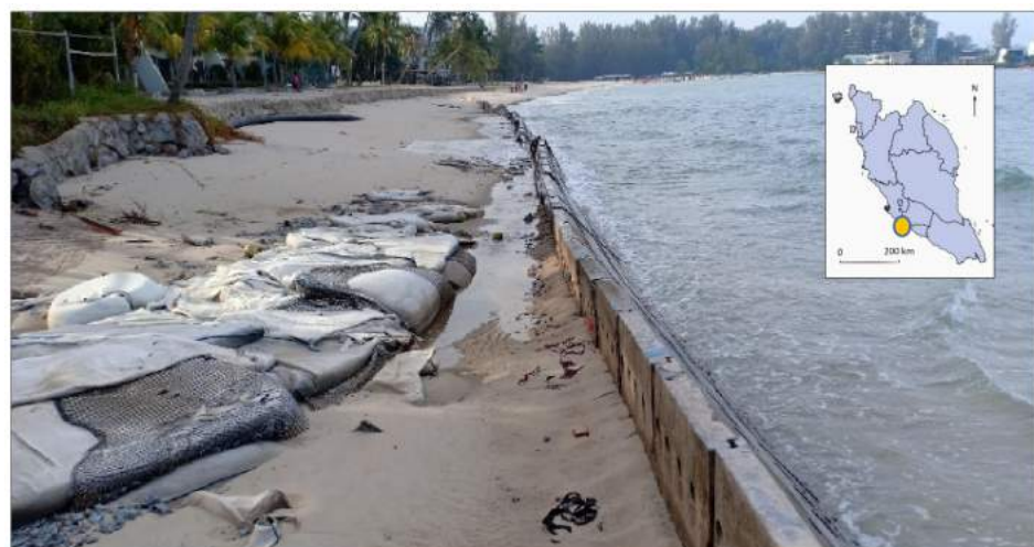
Figure 18. Damaged geotextile-tube replaced with concreted structure protection [110].
