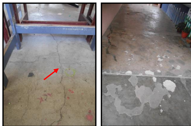
Figure 4. Photos of slab defect.
