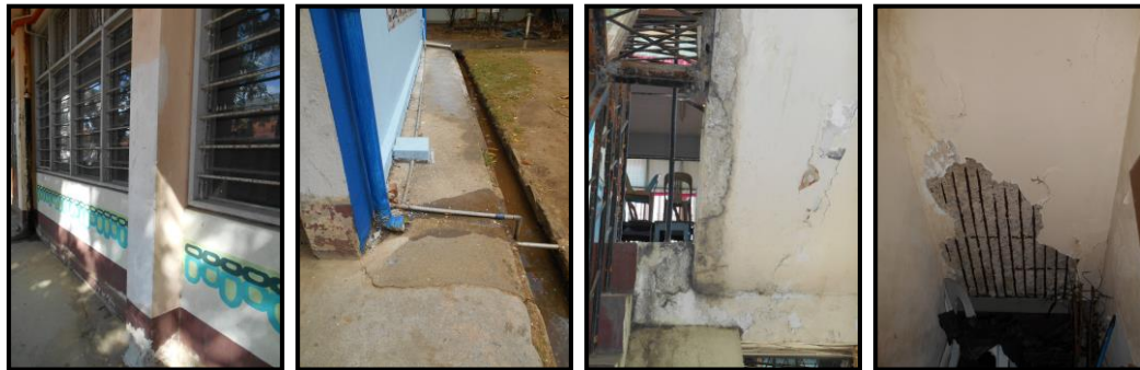
Figure 3. Photos of settled apron and staircase defect.
