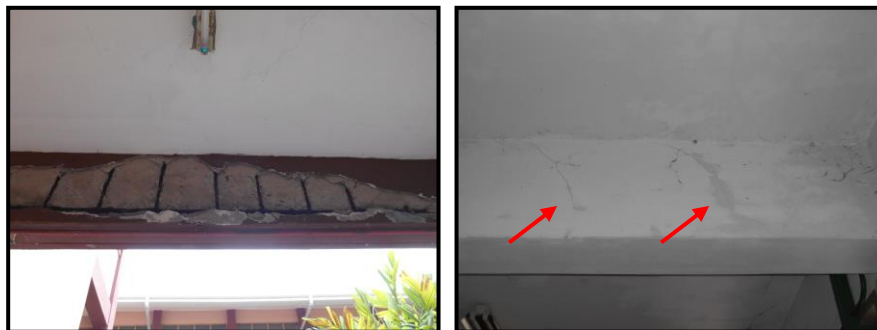
Figure 5. Photos of beam defect.
