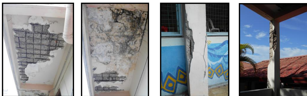
Figure 2. Photos of ceiling and column defect.
