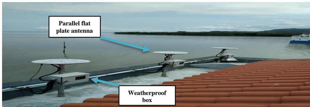
Figure 1. Three parallel flat plate antennas with weatherproof boxes
