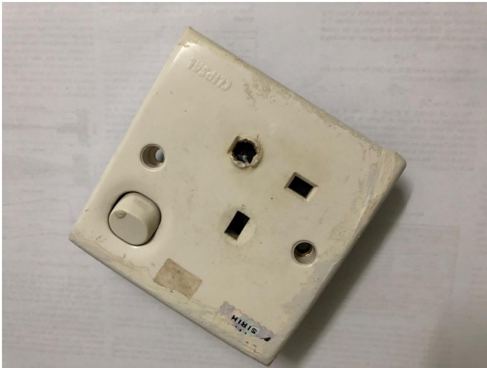
Figure 1.1: 3Pin Plug Damage by Arcing
