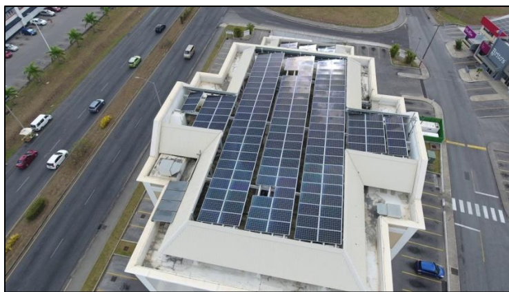
Figure 1.3 Solar PV mounted on roof top building
