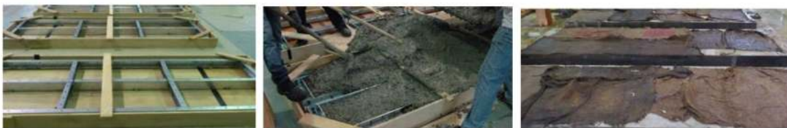
Figure 6. Foamed concrete slab with cold-formed steel as reinforcement [80]. Reprinted with permission from [80].
