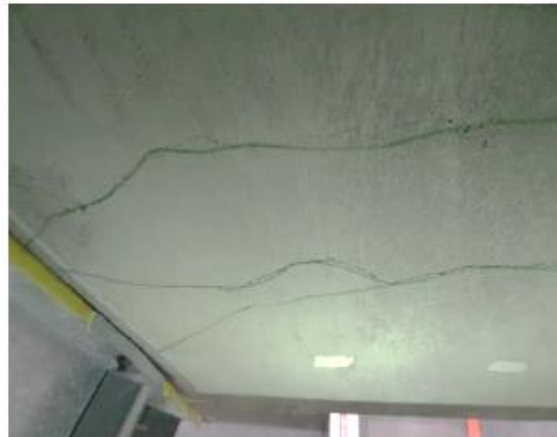
(b) Transverse cracks underneath slab
