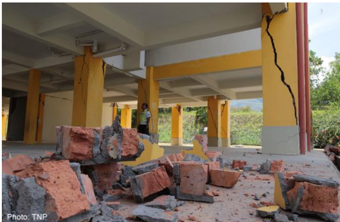
Figure 1.2 Crack of columns of a building after the earthquake (Vanar, 2015)
