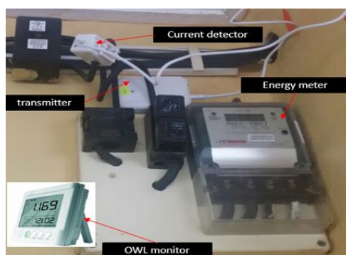
Figure 1. Photo of OWL installation at energy meter (TNB meter)
