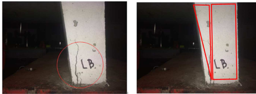
Figure 9. (a) Crack at inner part of USSP web (b) Crack only occurred in triangle area
