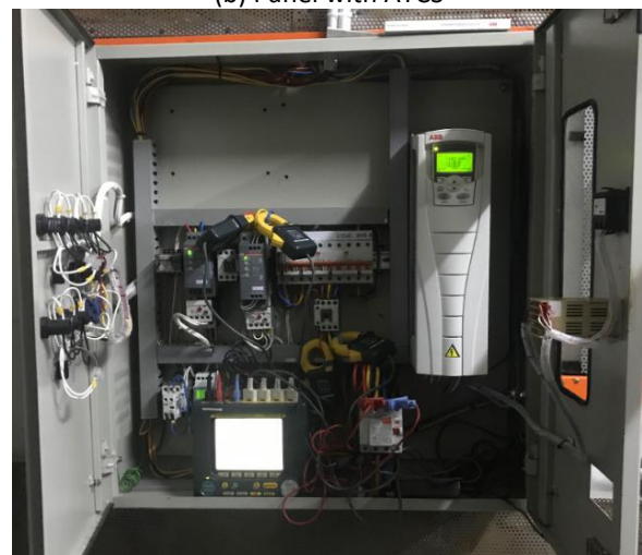
(d) Inside the panel after installation of ATCS with inverter and soft starter
