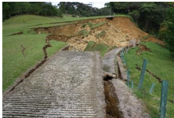
Figure 1. Ground failure after an earthquake hit Ranau, Sabah.
