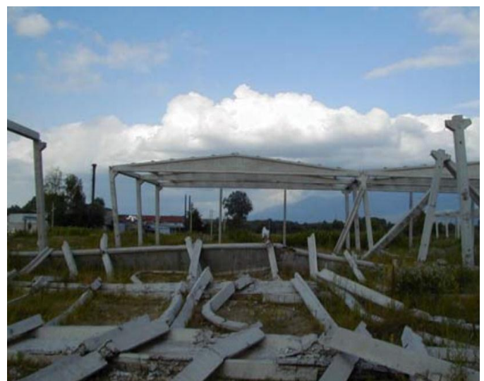
Fig 2 Seismic induced damage to precast industrial buildings in Turkey (reprinted from [36] )
