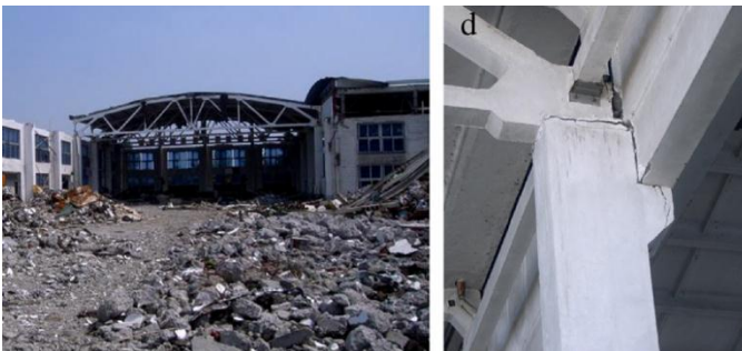
Fig 4 A damaged precast industrial building in China (reprinted from [38], Copyright Elsevier, 2009)
