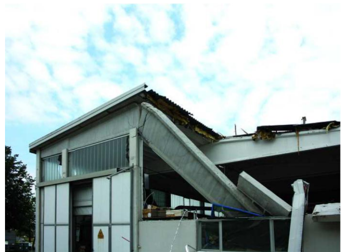
Fig 1 A damaged industrial precast building after Emilia earthquake in Italy (reprinted from [34], Copyright ASCE, 2001)
