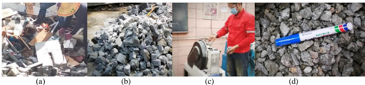
Figure 3. (a) Concrete waste breaking, (b) Demolished concrete, (c) Crushing the concrete, and (d) Recycled concrete aggregate.
