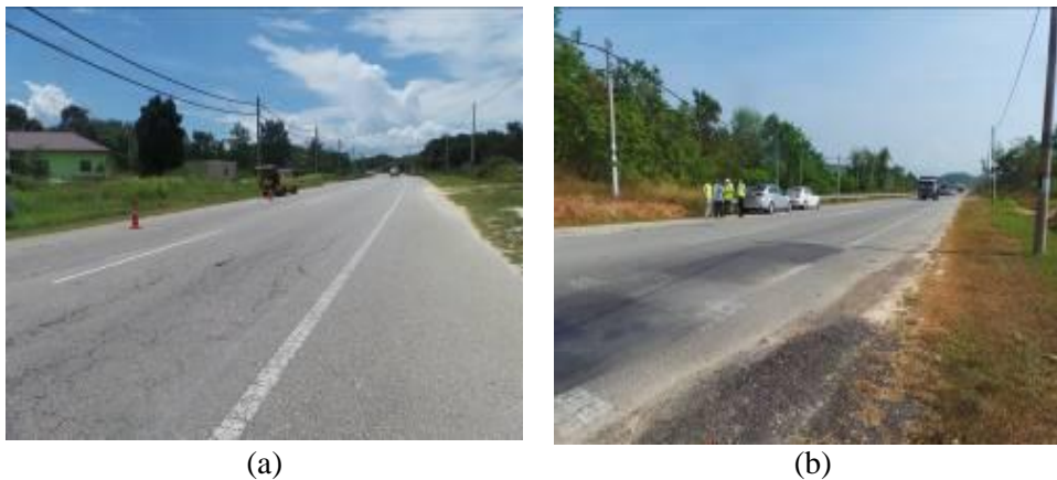
Figure 2. The condition of the existing road. (a) conventional asphalt section before construction and (b) cup lump modified asphalt section before construction.
