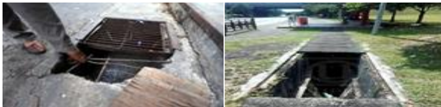
Figure 3. Vandalism of cover slab which cause safety issue for public.
