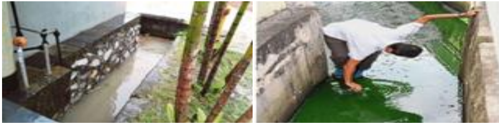
Figure 2. Stagnant water in the drain cause by unsmooth flow, which create the fertilization mosquitos.
