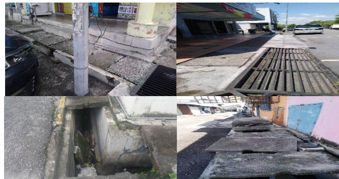
Figure 4. Existing conditions before eco-composite drainage systems are implemented in Shah Alam, Selangor.
