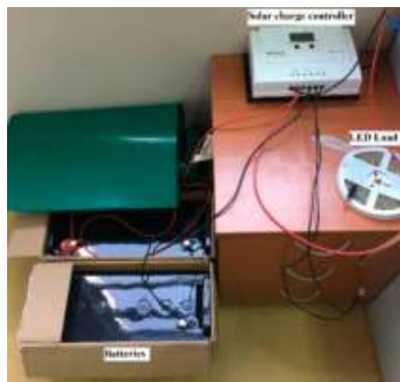
Figure 5. Batteries, LED load, and solar charge controller placed inside the G3 building in UTM, KL.
