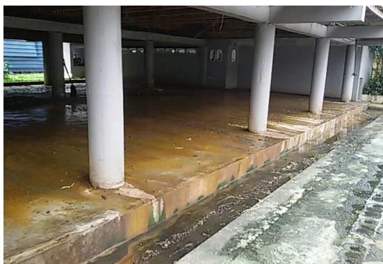
Image 4.6: Shelter Waste Management
