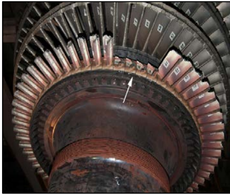
Failed gas turbine engine, [4]
