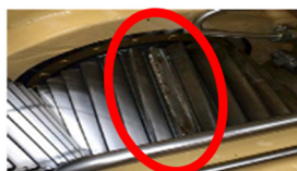
Fig. 10. Vestas V90 Hansen gearbox fault condition
