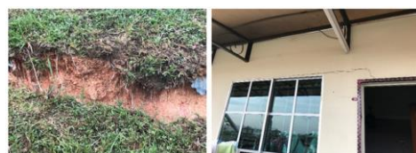
Figure 3. Images of landslide and building cracks at the study area
