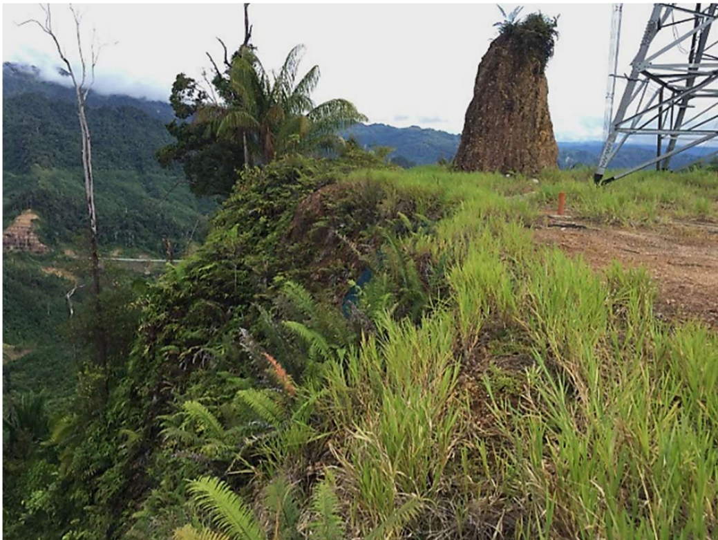
Figure 1.4 Slope failure adjacent to transmission tower
