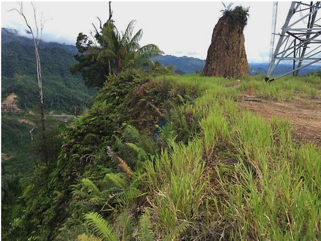
Figure 1.4 Slope failure adjacent to transmission tower
