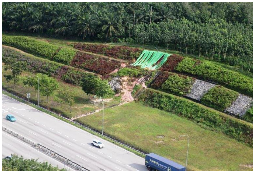
Figure 1.1 Overall view of failed slope at KM424.80 South Bound
