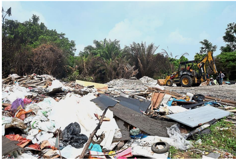
Figure 1.1: One of the four illegal dumpsites in Kampung Laut, Skudai.
