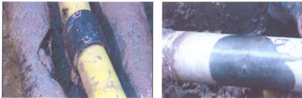
(a) Ruptured pipes at incident site
