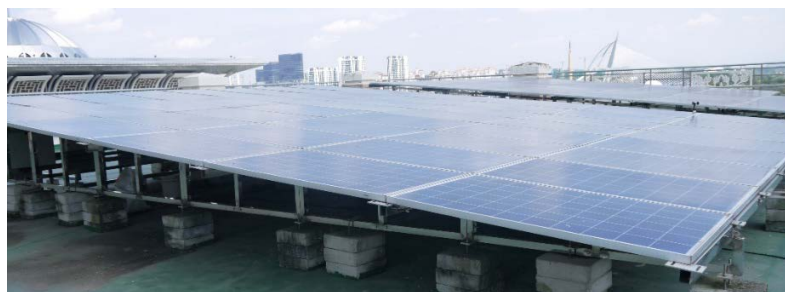
Figure 1.2 The PV Panels are installed at BHEUU
