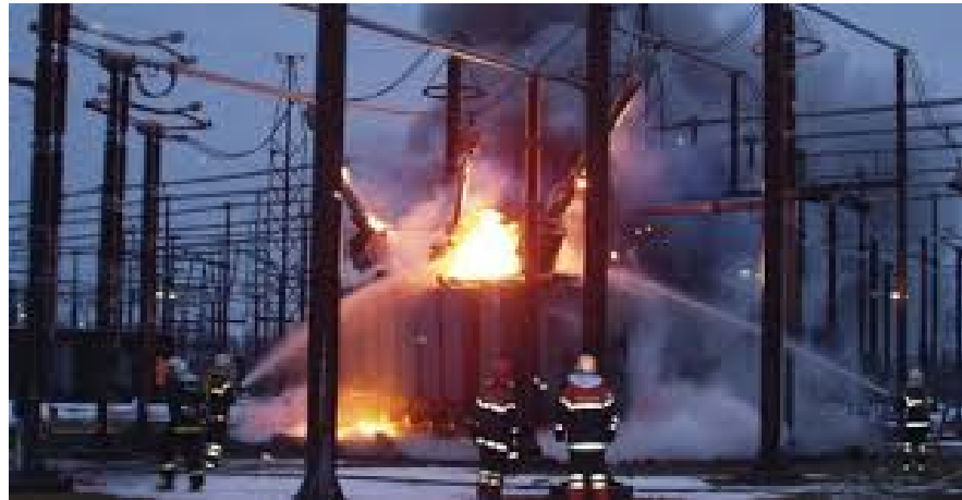
Figure 1.3: Insulation Failure Lead To Equipment (Transformer) Loss
