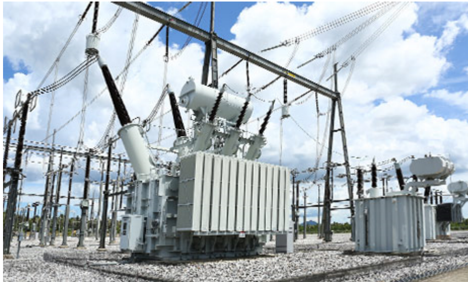
Figure 1.1: Typical Power Transformer In Power System Network
