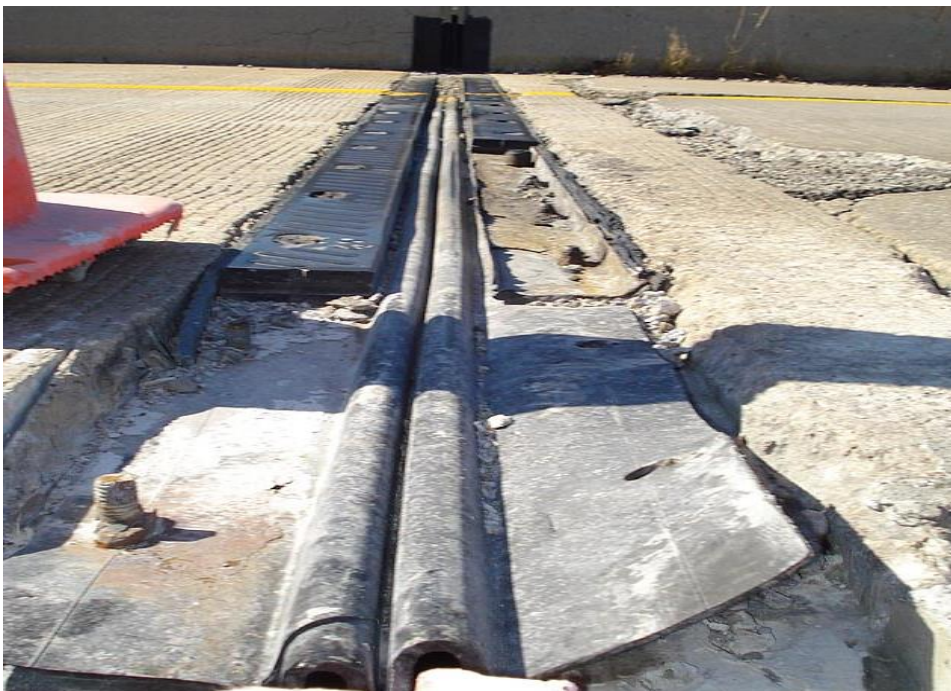
Figure 1.3 Dangerous expansion joint failures (Emseal Infrastructure & Civil Products, 2014)
