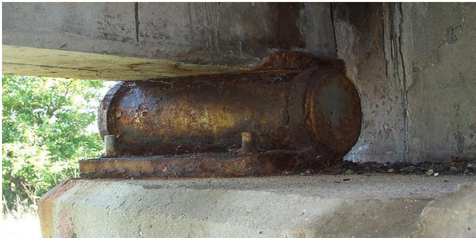
Figure 1.5 Corrosion of bridge bearing (Michel et al., 2010)
