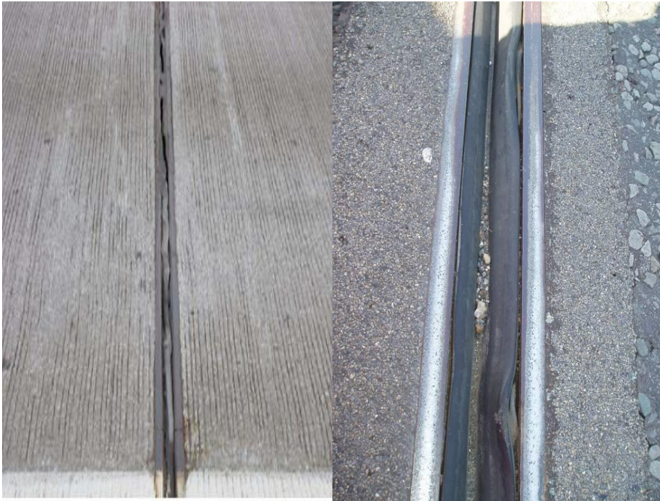
Figure 1.2 Expansion joint failures (BadwaterJournal.com, 2011)
