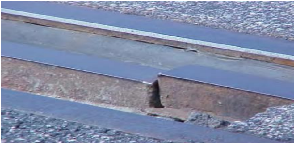
Figure 1.4 Dangerous expansion joint failures (Harry, 2006)
