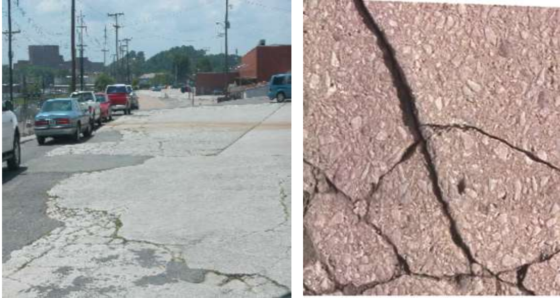
Figure 1.1. Image showing road cracking (Yu et al, 2005).
