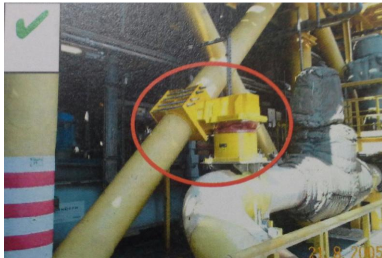
Figure 1.4 Viscous damper added to reduce the vibration level of piping system (Energy Institute, 2008)
