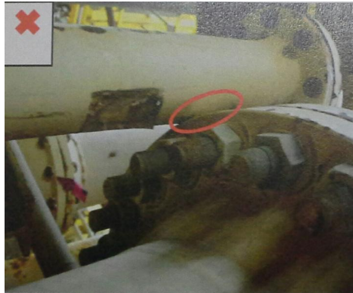
Figure 1.2 Fretting damage caused by clash between pipes (Energy Institute, 2008)
