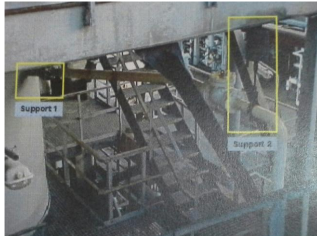
Figure 1.3 Additional support in piping system to brace the piping structure (Energy Institute, 2008)
