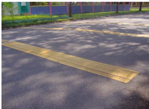
Figure 1.1 Typical TRS in Malaysia
