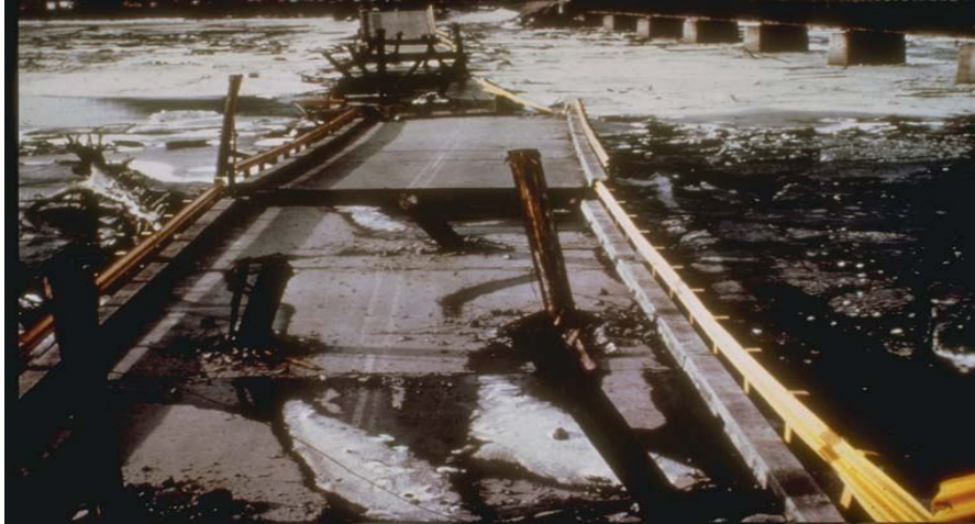
Figure 1.1 Collapse Twenty nine mile River Bridge supported on Timber Piles in the 1964 Alaskan Earthquake (after Meymand,1998)
