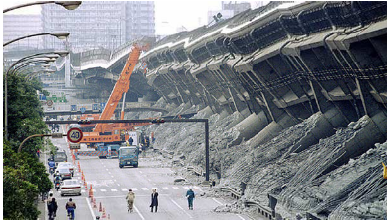
Figure 1.5 Higashi-Nada Viaduct collapse in the 1995 due to Kobe earthquake (Chen and Duan, 2003)
