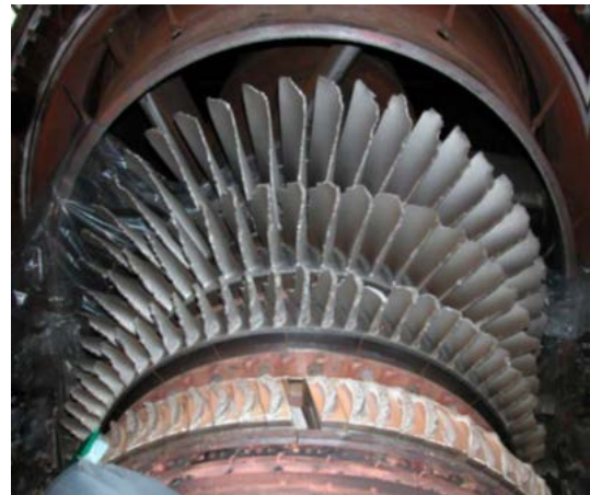
Broken blades at different stages [11]
