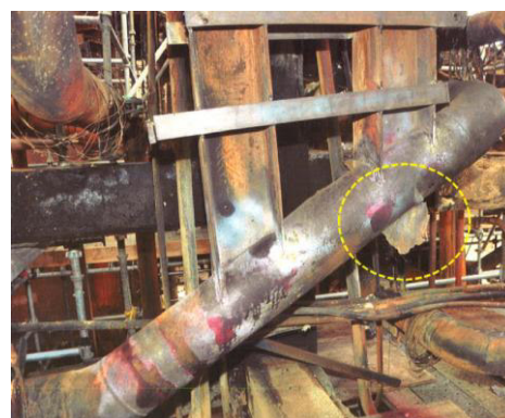
Figure 1.9 Evidence of sulfidation corrosion in the ruptured pipe
