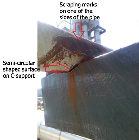
Fig. 4. Actual pipe portion resting on C-support.
