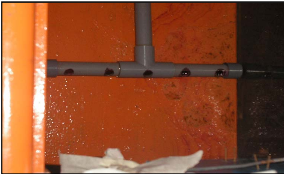
Photo 3.3: PVC pipe with 5 holes and 12 mm diameter each multi-port diffuser.
