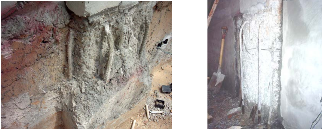
Figure 1.1 : The damage to the column
