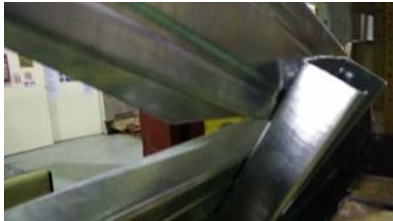
(a) Failure on connection between the intermediate member and top chord
