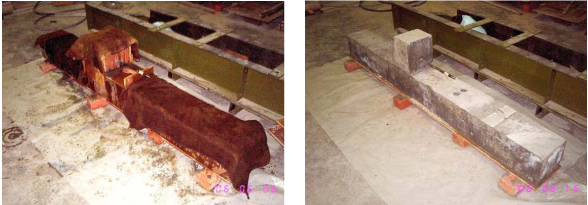
Figure 8 Preparation of precast column with corbel (specimen 4): formwork preparation, concrete casting, curing and the completed specimen (from left, clockwise)
